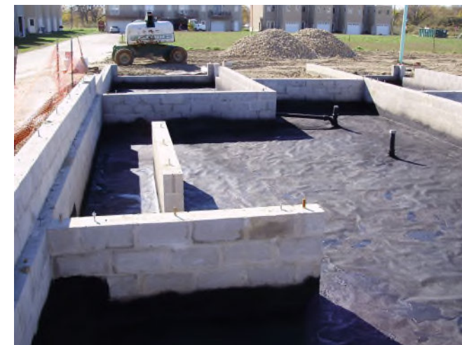
Example of a passive vapor barrier at Siena Place
