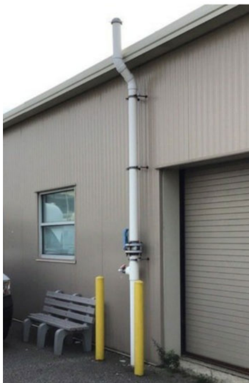
Example of passive vapor mitigation system (PHA Building shown)
